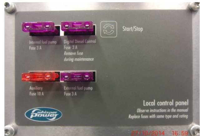
Figure 7: Local control panel
